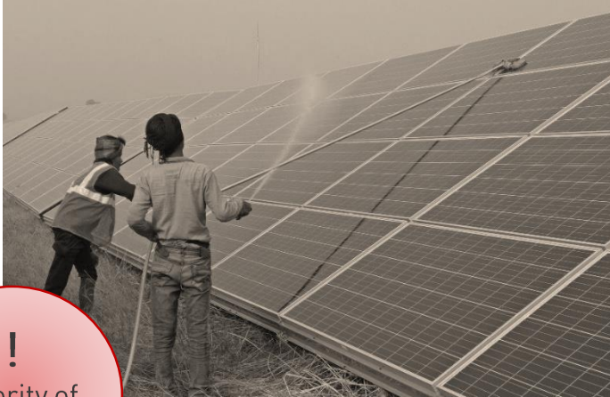
Manual wiping with water hose
